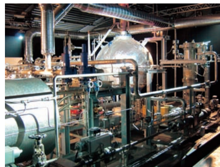
Pressure storage vessel, pumps and pipework
